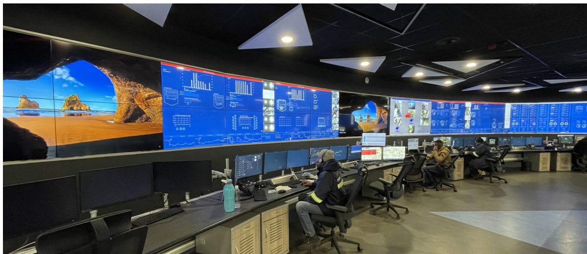
The completed iROC operations floor: a continuous video wall of 84 panels serving 21 operator stations.
